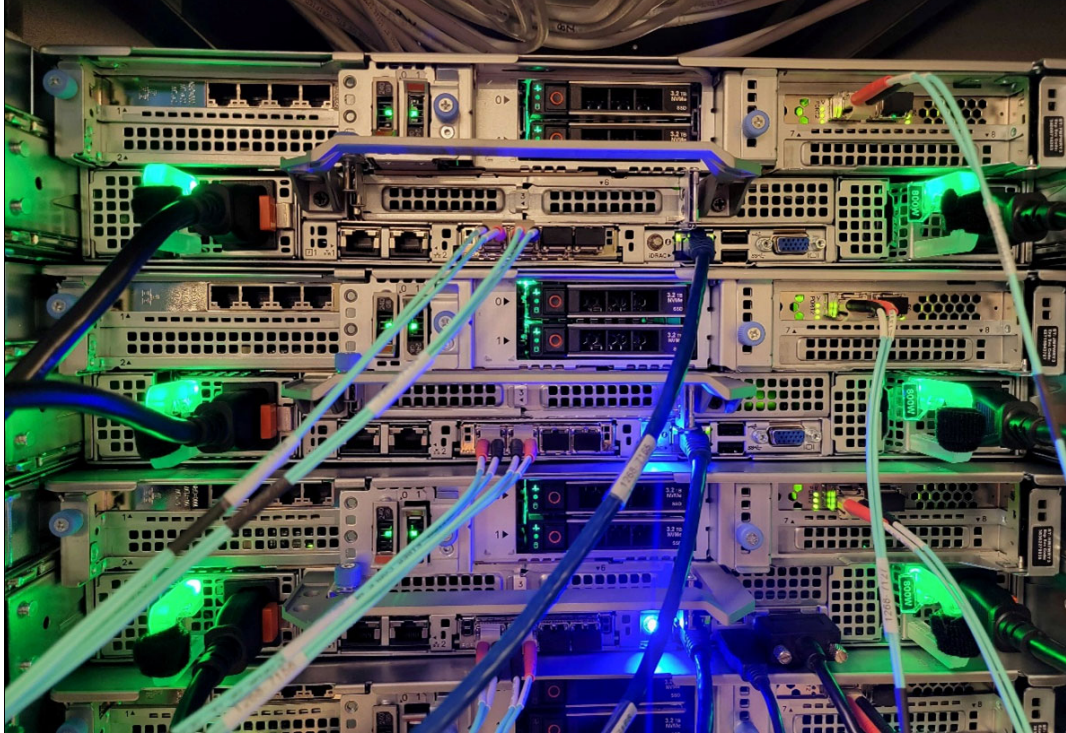
Figure 3-16 IBM Storage Ready Nodes management and network and optional FC adapter access via the rear of the cabinet
