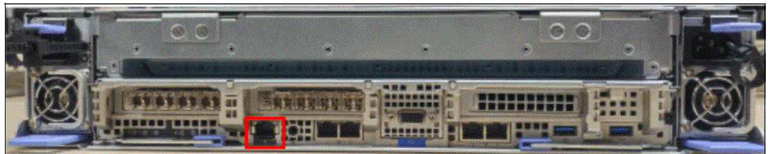
Figure 2-8 Technician port IBM SAN Volume Controller 2145-SV2
