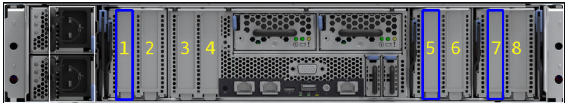
Figure 8-4 Dual Port 100 GbE adapter placement on SAN Volume Controller node SV3
