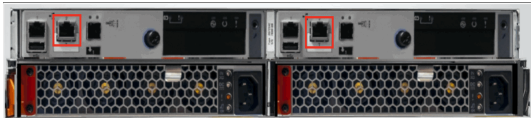
Figure 3-4 Location of the technician port on IBM FlashSystem 5010
