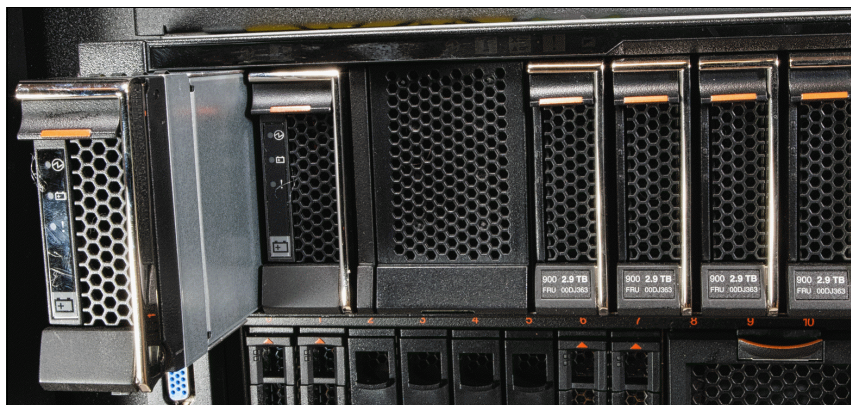
Figure 3-19 Flash enclosure battery module 1 partially pulled out
