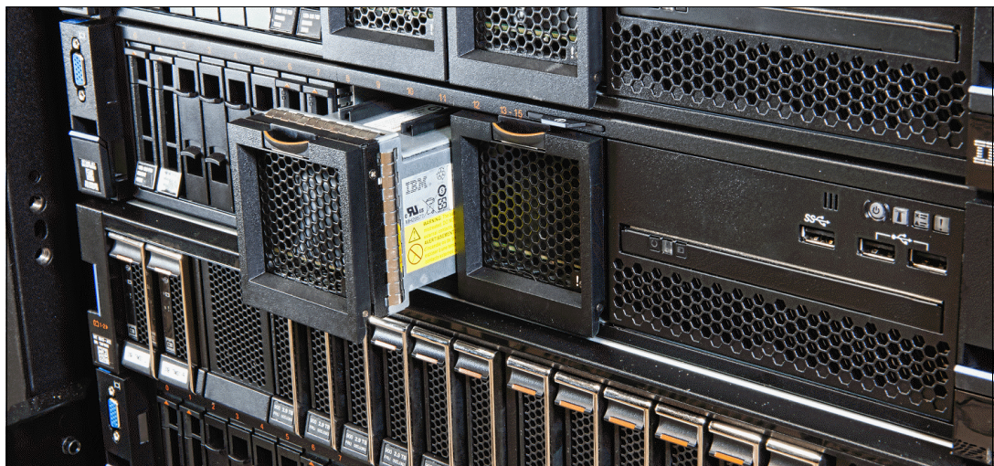
Figure 3-7 Grid controller with a battery that is pulled out
