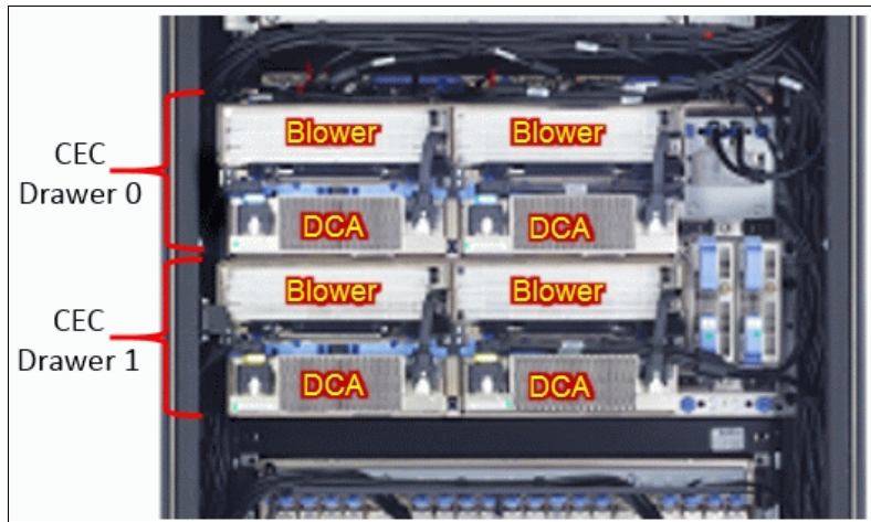
Figure 2-11 Redundant DCAs and blowers for CPC drawers
