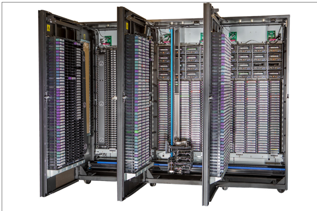
Figure 1-5 L55/D55 frame internal view
