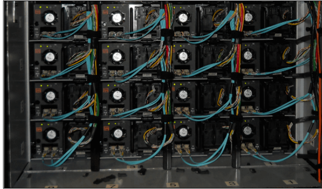
Figure 1-34 TS4500 drive bay
