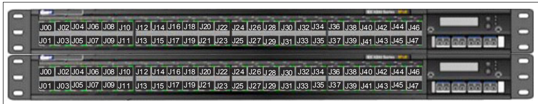
Figure 7-7 Two 1000BASE-T TOR switches (INMN)
