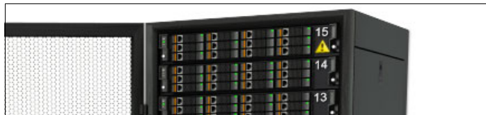
Figure 7-23 Module temperature threshold exceeded
