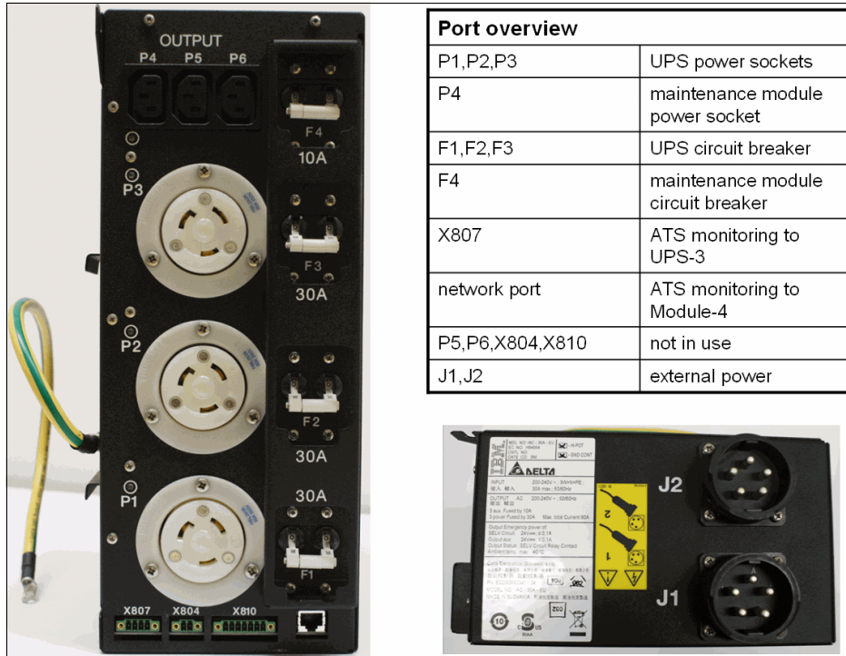
Figure 3-11 Automatic Transfer Switch
